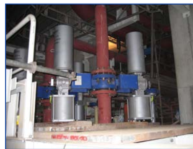
ESD turbine trip
